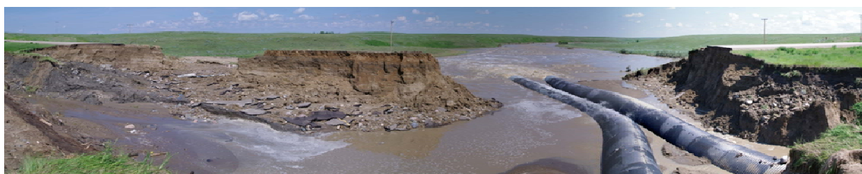
Figure 3 – Damaged roadways and culverts, looking north.
