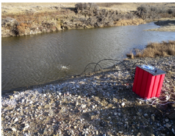
Figure 9 – Aeration system to prevent ice forming in temporary fish habitat.
