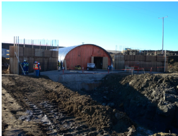
Figure 6 – Hoarding the culvert to prepare for granular backfill placement in winter conditions.
