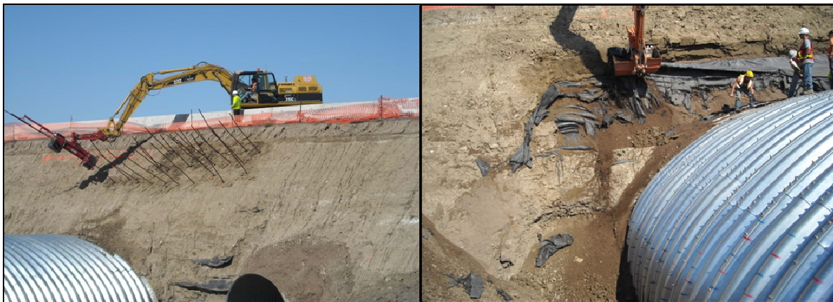
Figure 10 – Installing soil nails to strengthen westbound lanes for excavation around 2010 arch culvert construction.
